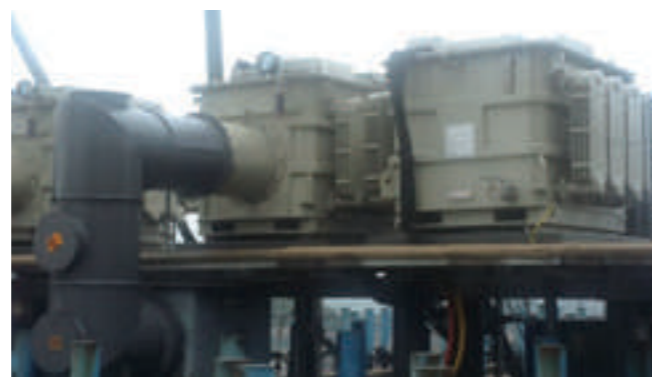
Micro Pulse System in coal power plant in Hunan province, China
